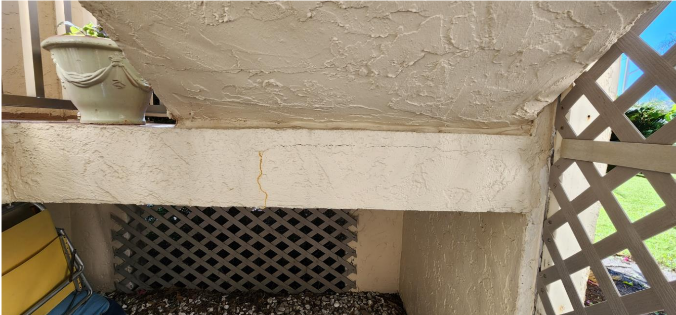
MINOR CRACKS BELOW THE STAIR
