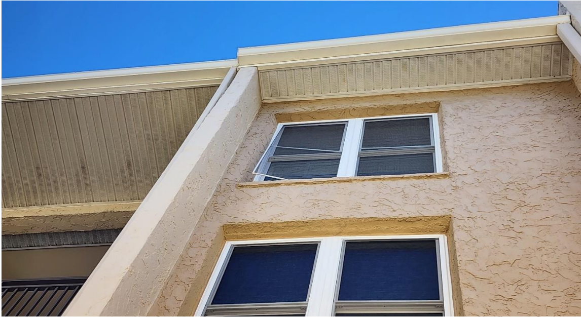
LOOSE WINDOW SCREEN
