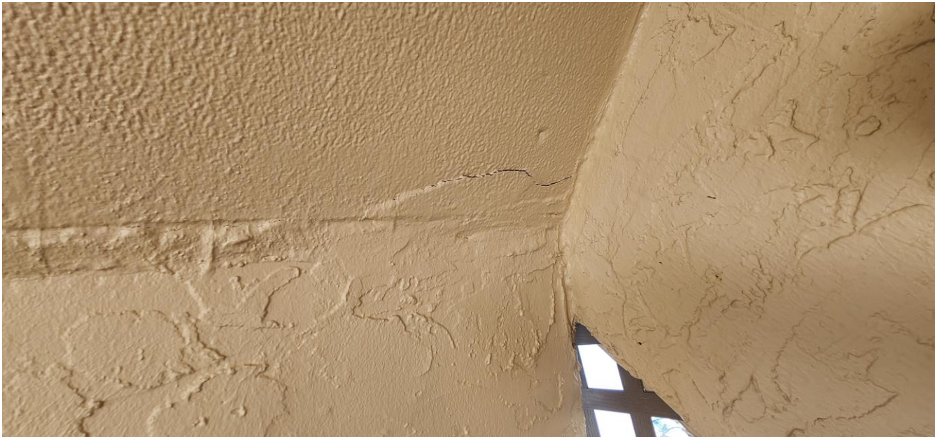
MINOR CRACKS BELOW THE STAIR
