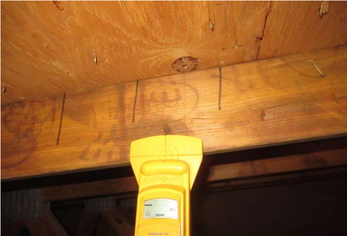
Nail location verified
